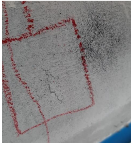
Figure 9 : Circumferential crack field SCC from TRAPIL field investigation
