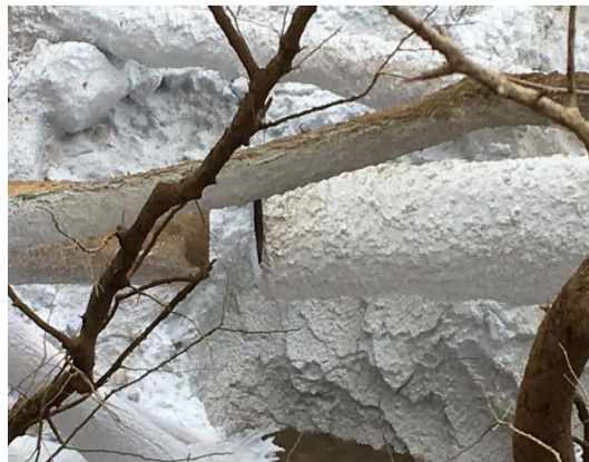
Figure 8 : circumferential fatigue crack in a CO 2 transport pipeline due to ground movements [6]
