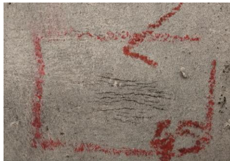
Figure 10 : Axial crack field SCC from TRAPIL field investigation
